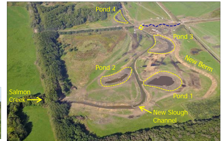
Construction of 4,205 feet of new slough channel and four fresh and brackish water ponds were completed 2011.
