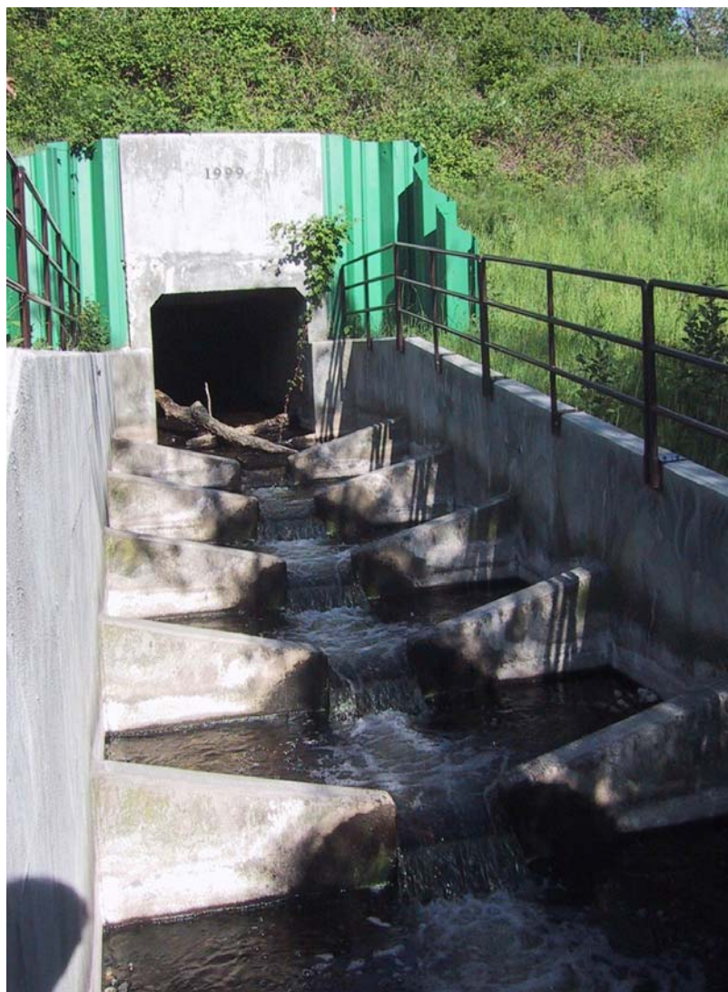
Figure XII-48. Fisher Creek pool-and-chute fishway at low flow.
