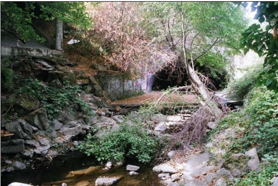
Figure 1 - Outlet of the Lansdale Avenue Crossing on San Anselmo Creek (2006). The outlet is a concrete single radius arch approximately 15-ft high and 30-ft wide with a 36 foot long concrete apron perched approximately 3 feet above the downstream channel.
